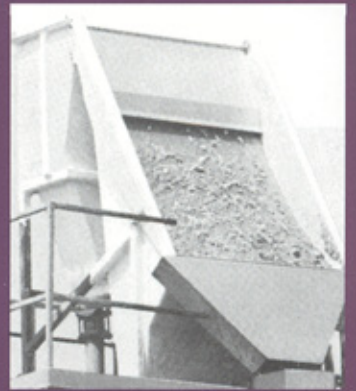
Wastewater Screening For Carrot Processor
